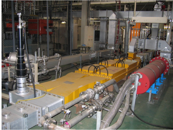
RF high power system
